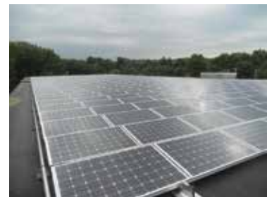
Solar Panels to trap solar energy
